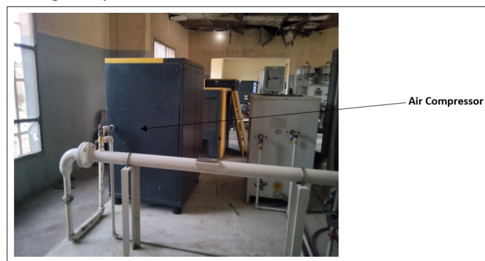
Figure 1: ASD 32 Air Compressor (Disc Pressure 8bar, Power 185kw)
