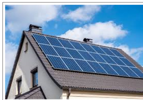
Figure 6: Solar Panels on a House
