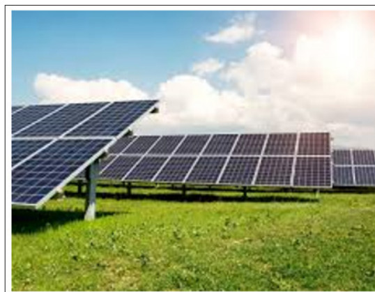
Figure 7: Solar Panels in a Field
