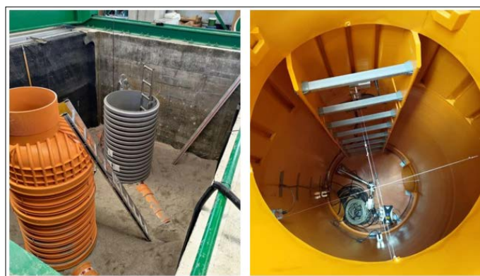
Figure 2: Testing layout, instruments in the manhole
