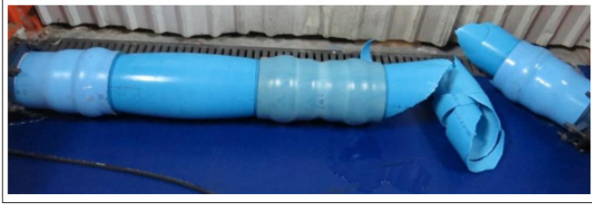
Figure 4: Pipe Burst Away from the Joint.
