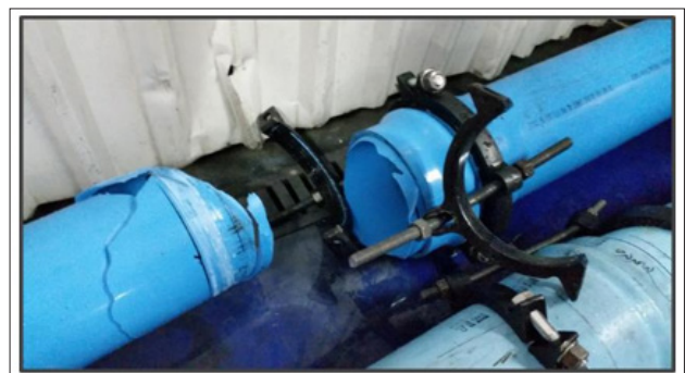
Figure 1: Brittle Failure of Spigot At 400psi
