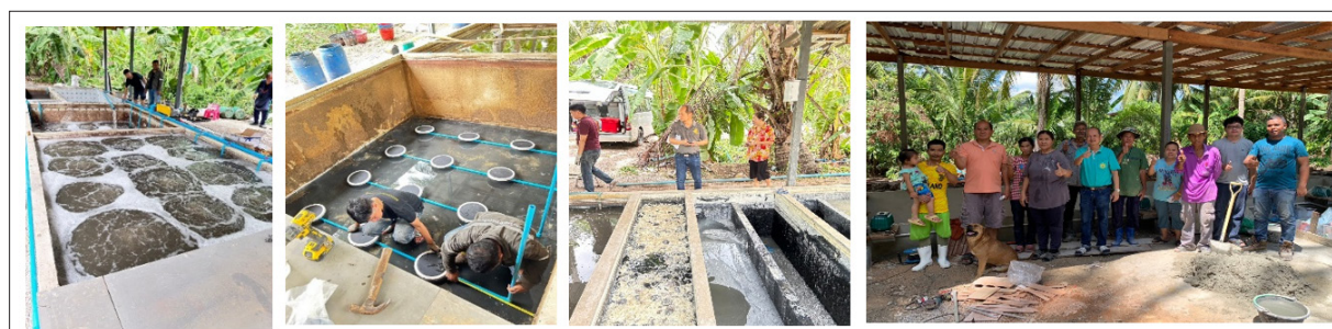
Figure 3: Installation and Operation of Pilot Scale Wastewater Treatment System
