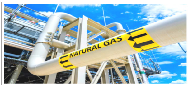
Figure 16: Natural Gas Processing Plant to CNG
