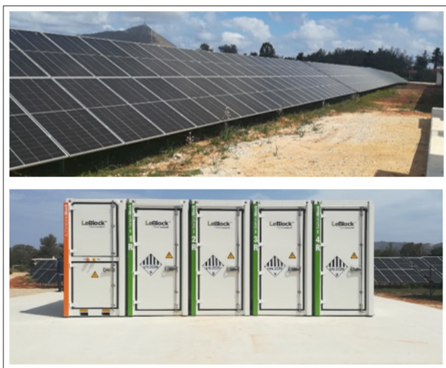
Figure 10: The Lighthouse Project in Chania Airport: PV panels and BESS (Source: HEDNO S.A.).
