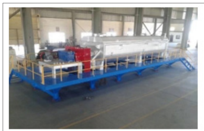
Figure 4: Paddle Dryer Plant
