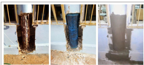
Image 7: Shows the process of corrosion column reinforced concrete repair [17,18].
