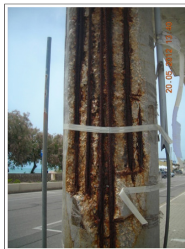
Image 5: Shows Iron rusts in concrete
